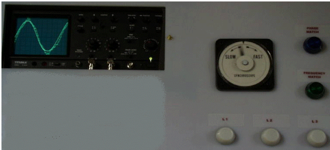
Figure 27: Successful Synchronization of the Generator to the Reference Bus
